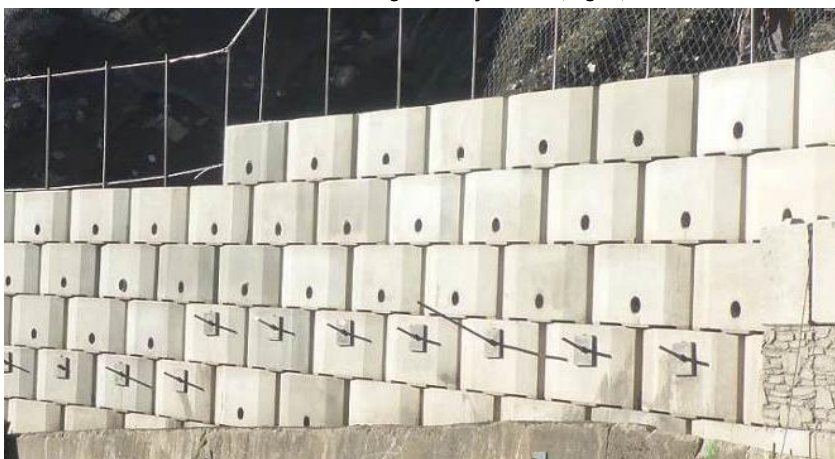
Figure 4: View of the structure with steel bares and net on the top
