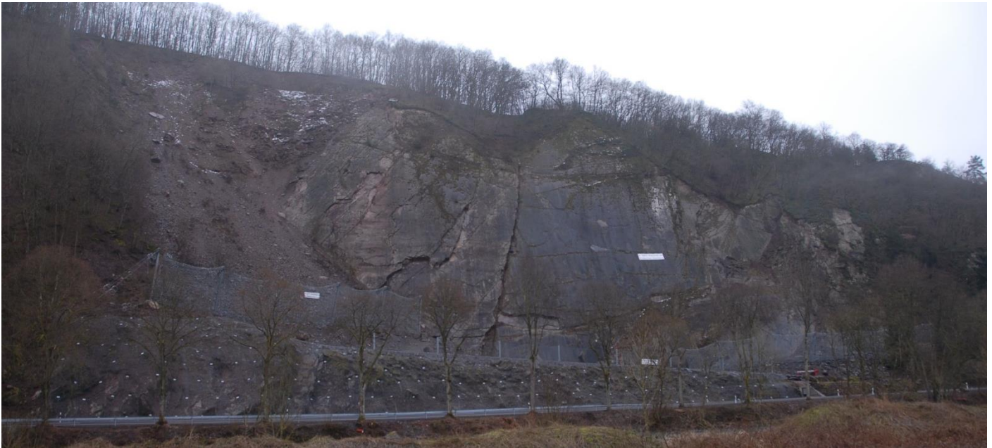
Figure 2: Overview of the measures against the rockfall hazards at the former quarry Carriere de Michelau
