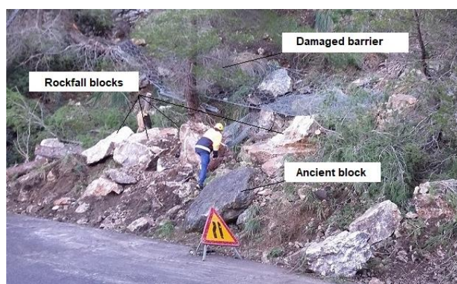
Figure 1: Formentor rockfall of 30 th January 2017
