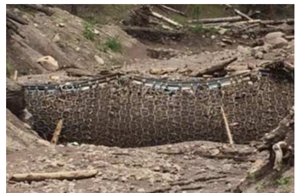
FIG3: Filled Debris Flow Barrier at a neighbouring Pueblo.
