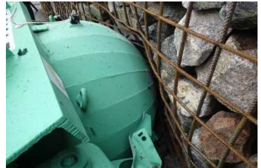
Figure 4: Deformation of the facing after the first impact at 400kPa
