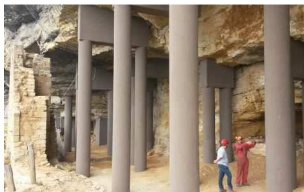
Installation of 9 concrete gantries for final supporting, formworks with tubular cardboard - on site concrete mixing
