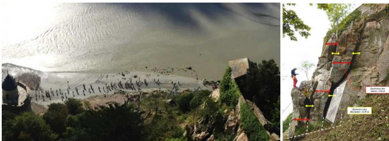
Figure 1 and 2 : Big issue with hundreds of tourists crossing below unstable rock mass
