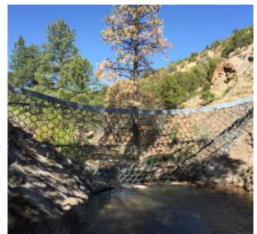
FIG2: Debris Flow Barrier in Nambe Pueblo
