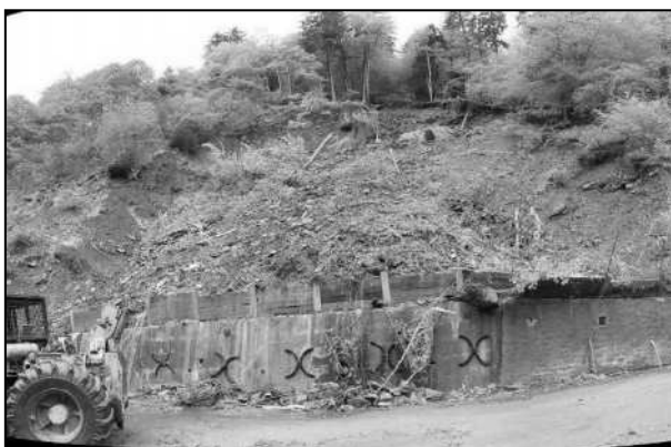
Figure 1: Sight of the rockfall – 2 May 2015
