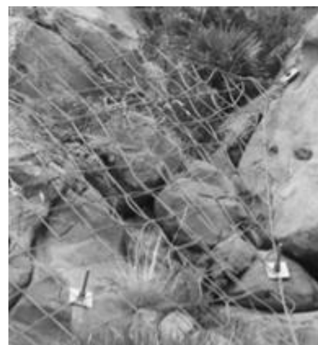
Figure 1: Example of stuck block stabilization
