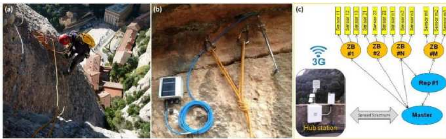
Figure 2: WSN in Montserrat: a) installation works; b) ZBLogger for a crackmeter; c) scheme of the network from sensors to datalogger in the hub station through ZBLoggers, master node and repeaters
