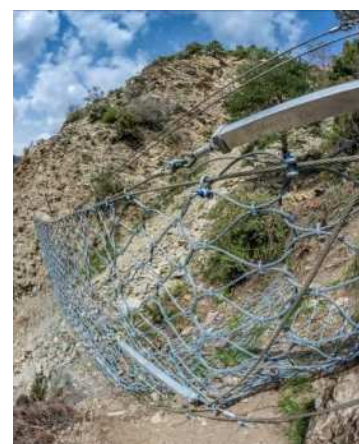
Figure 2 and 3 : example of wire rope barrier against debris flow
